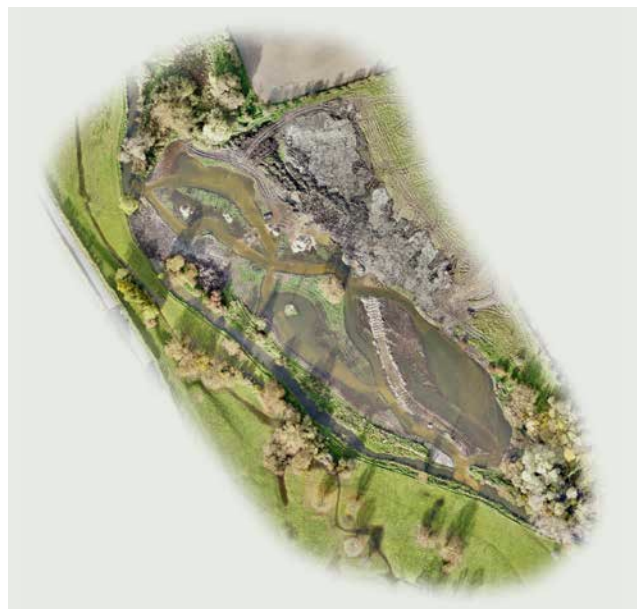
Figure 3. Completed new channel and wetland features immediately post construction, 9 November 2023. Photo credit: Kev Morris.
