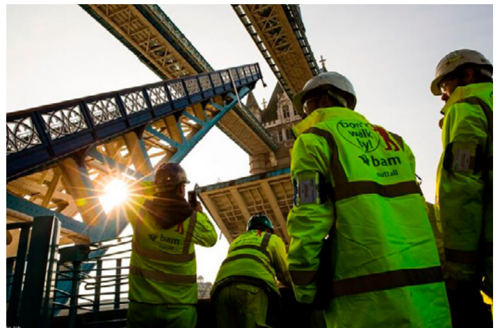
THERE WAS A TOTAL OF 84 BRIDGE LIFTS DURING THE CONSTRUCTION WORKS, AND PEDESTRIAN ACCESS REMAINED OPEN
